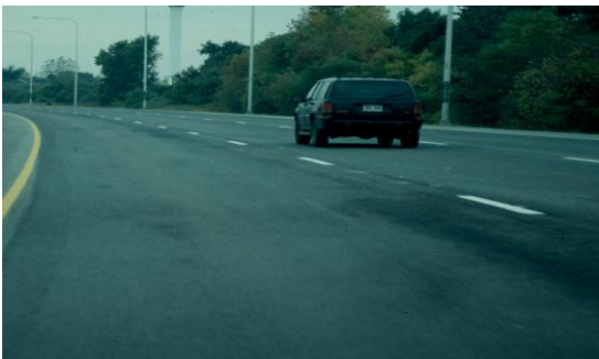
End of Load Segregation
