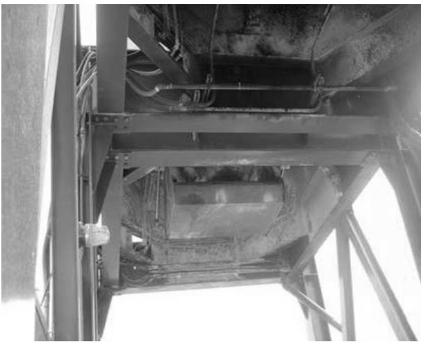
Silo Discharge Gate
