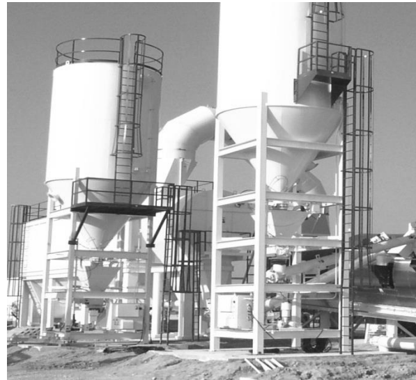
Dust storage tanks w/weigh pod
